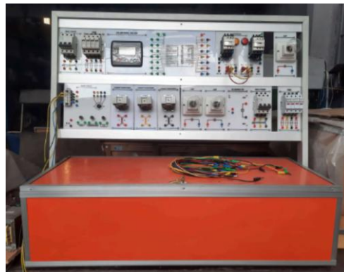
Figure 5. Photo of the industrial-based AMF power system training unit installation.
